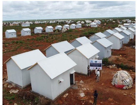
UNHCR completed the construction of 70 semi-permanent shelters in Barwaqo-2 Durable Solutions Site, Baidoa. © UNHCR
