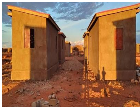
Ongoing construction of permanent shelters at the Harwanag Site in Adado. © NRC
