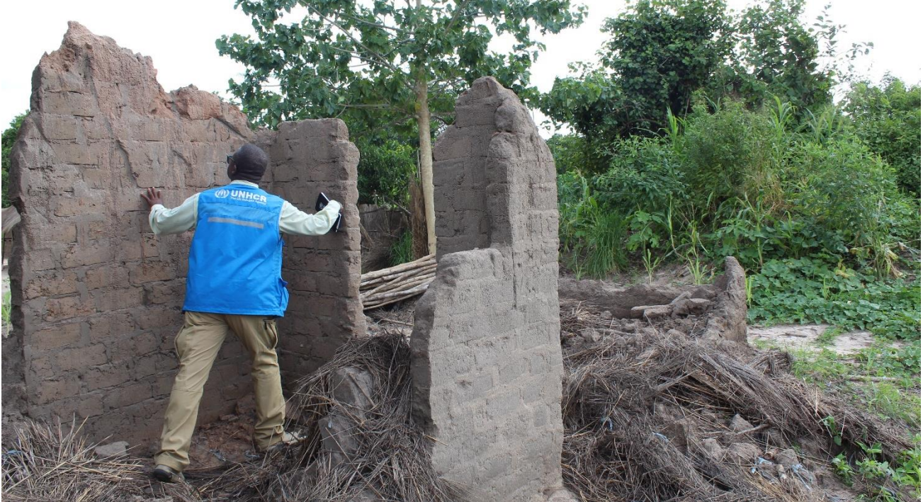
Assessment of completely damaged shelters by cyclone Jude in Memba District, Nampula Province. ©UNHCR/Eduardo Burmeister.
