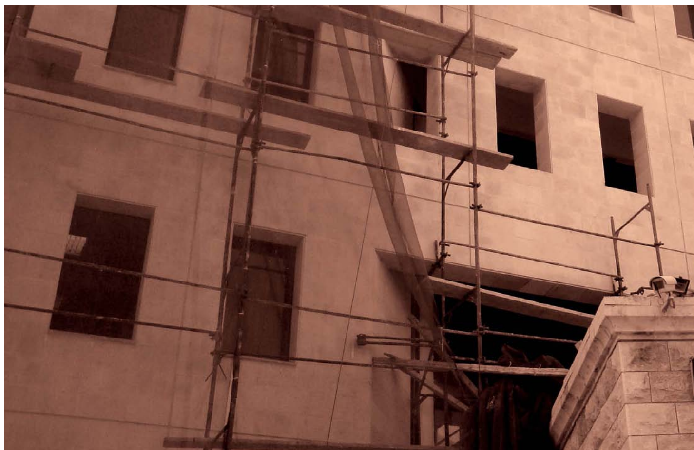
Picture 18 In addition to the market incentives, the Central Bank implements energy efficiency measures in its own premises
