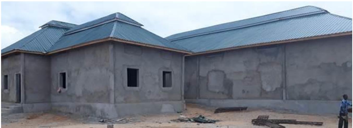
Construction of the police post at the new shelters, Kismayo ©UNHCR/ 31 August, 2018.
