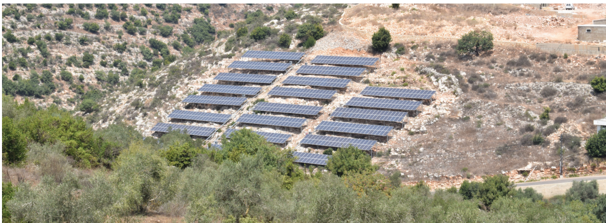
Figure 2: 250 kWp system implemented at Kabrikha, South Lebanon
