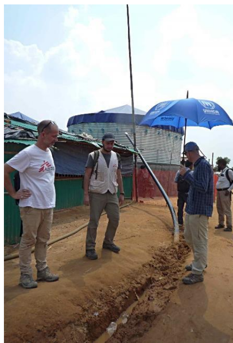
Pipes are being laid to distribute chlorinated water from the reservoirs to tap stands in Camp 1E settlement, Kutupalong, in early October. ©UNHCR/I. Susanti
