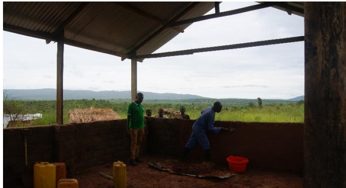
A hangar under construction in Sango Malumbi, Tanganyika Province to store adobe bricks made by returned IDPs © UNHCR/Stenbock-Fermor
