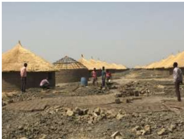
Durable shelters called 'tukuls' in construction in Al Jameya camp in White Nile State. Photo credit: UNHCR, February 2019.
