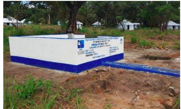
A borehole in the new Bele settlement. © UNHCR
