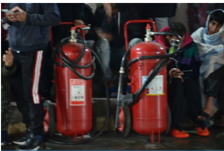
Fire extinguishers in TRC Bira © IOM BIH 2020
