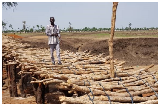
UNHCR and ACTED rebuilt this essential bridge in Upper Nile after it was destroyed by flooding. © UNHCR/Joseph Wani
