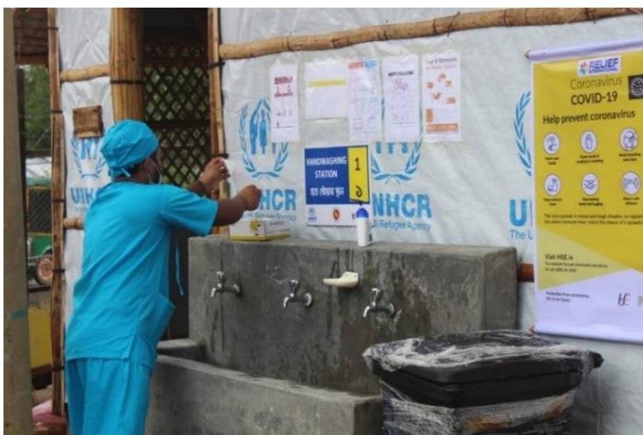
Handwashing facilities at UNHCR’s Severe Acute Respiratory Infection Isolation and Treatment Centre in Ukiya. © UNHCR/Louise Donovan
