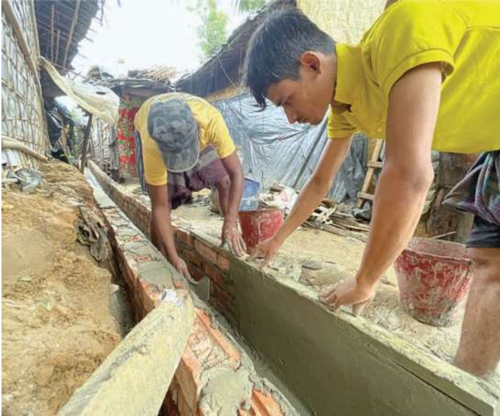
Community-led projects are identified through consultations with the community and coordination with relevant actors. Projects included construction and repair of pathways, bridges and stairs to facilitate safe movement in the camps, in particular through the monsoon season. The projects are identified and led by the Rohingya refugee communities with support from UNHCR partners. @UNHCR/Amos Halder
