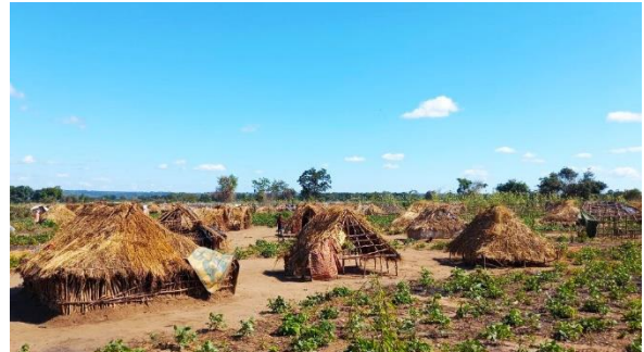
Shelters in urgent need of rehabilitation in Mueda District, Cabo Delgado. ©UNHCR/ Irene Matevu
