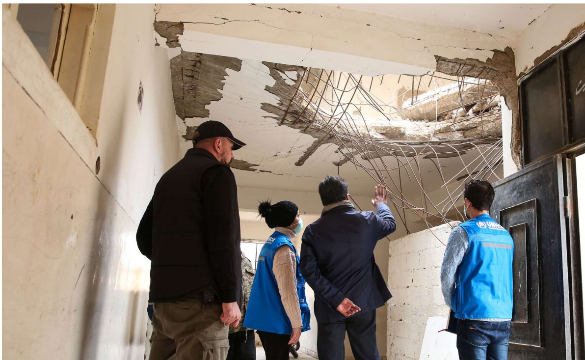
UNHCR's Representative in Syria, Sivanka Dhanapala visits a partially damaged school in Tishreen village in Al-Ashara sub-district, Deir-ez-Zor Governorate. UNHCR/V. Toumeh
