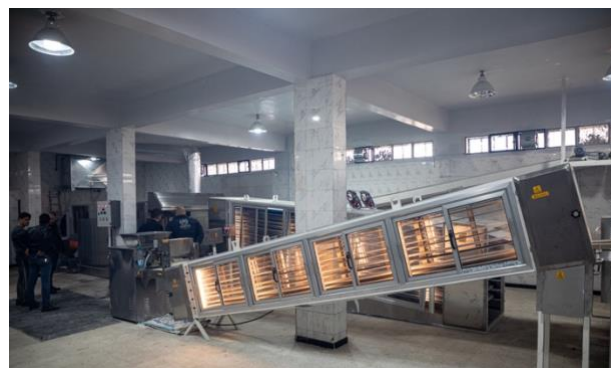
The repair of a bakery in Tal Hedia village, Aleppo Governorate, created job opportunities for many returnees. ©UNHCR/H.Maarouf
