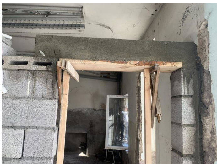
Reconstruction works are well in progress in Masis region, Ararat province. October 2023. © UNDP
