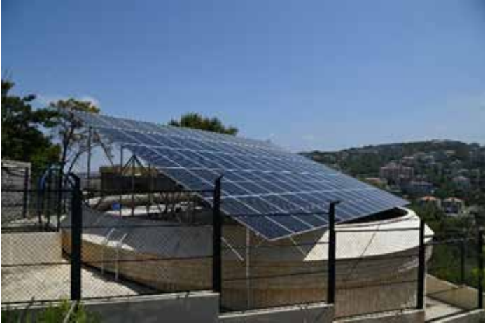
Solar panels installation for the Local water well catering for over 25,000 individuals in Choueifet city, in 2023.
