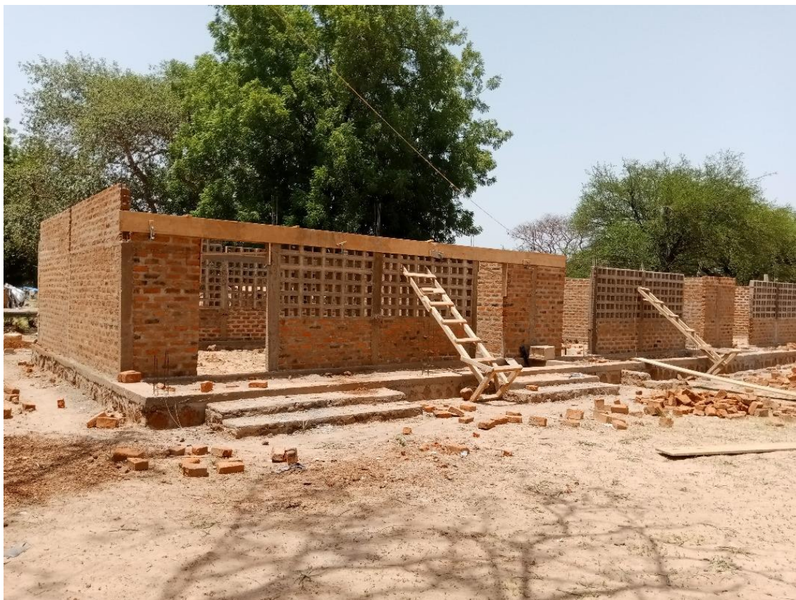
The construction of two school buildings with three classrooms each is underway in Birao, thanks to Education Cannot Wait's First Emergency Response Grant to the Central African Republic. ©UNHCR CAR
