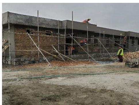
The Chilghor Comprehensive Health Center (CHC), under construction in Panjwayi's Chilghor village, will serve 19,000 locals, upon its completion.
