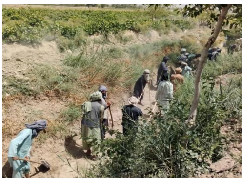
In 2022, the Salawat canal cleaning initiative provided jobs and benefited 6,867 locals, enhancing irrigation and economic stability. © ACHRO
