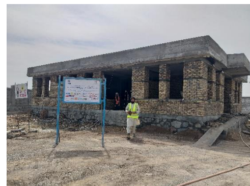
The Regwa Basic Health Center (BHC) project is currently under construction in the Regwa village, located in the Panjwayi district. Upon completion, the BHC is set to offer medical services to 15,000 People of Concern (POCs), of which over 51% are refugee returnees and internally displaced persons (IDPs). © WAW
