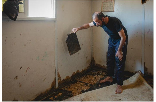
Most of the caravans in Zaatari camp have exceeded their designed life span of 5-6 years, and most families do not have the financial resources to consistently maintain their homes. ©UNHCR/ Shawkat Alharfoush
