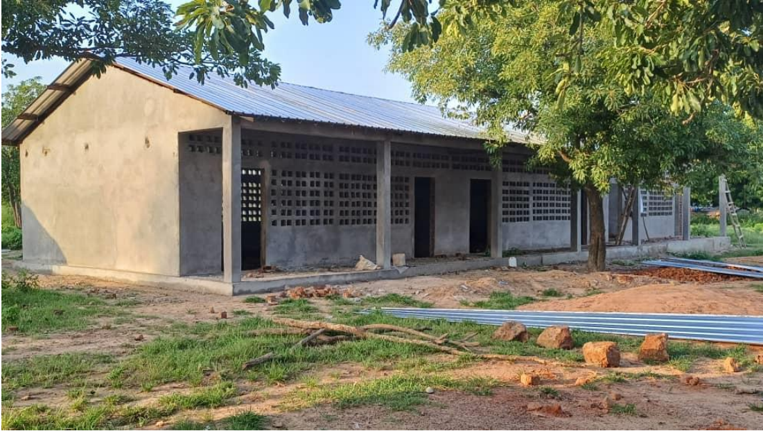
In Birao, work continues the construction of a building with 6 classrooms thanks to the generous support of Education Cannot Wait. ©UNHCR
