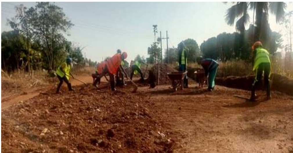
Work is ongoing to upgrade 2 km of Yumbe-Barakala-Bidibidi road to asphalt, employing refugee and host community casual labourers.
