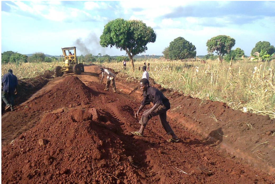
In Kiryandongo refugee settlement road works are underway to open up land plots for newly settled South Sudanese. ©UNHCR/ S.Koivogui
