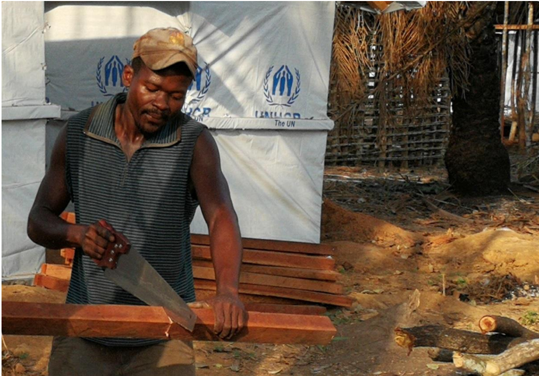
Construction of transitional shelters at the new Kaka site, Haut-Uele Province © UNHCR
