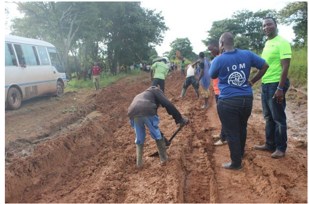
To ensure that the Government, UNHCR, sister UN agencies and other partners provide various services to refugees (including relocation), the Zambia National Service (ZNS) is clearing access roads in Mantapala Refugee Settlement ©UNHCR/B.Mulenga.
