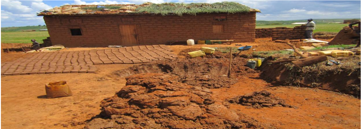
Figure 3 Excavating Soil for Moulding building blocks; an example of Human made wetland
