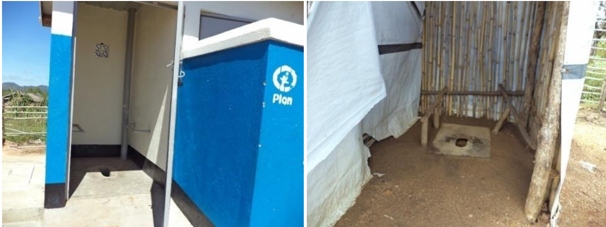
Latrines with provisions for CWD
