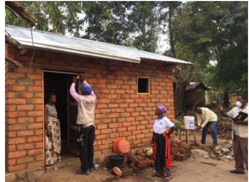
Finalization of a shelter in Kazimia, Fizi Territory, South Kivu Province. © AIDES
