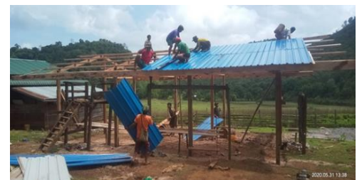
Construction of Early Childhood Care & Development Centre in Kayah State. Photo: UNHCR
