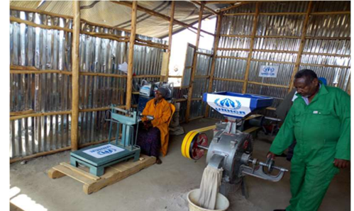
Newly installed grinding mills operational in Dire Dawa. Dawit Daricha/UNHCR Feb 2022
