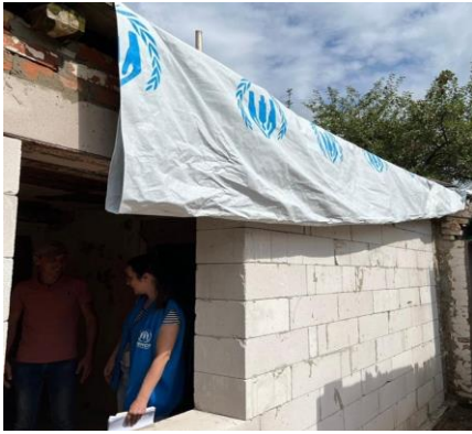
Repair works starting in Makariv in the Bucha district of Kyivska Oblast. August 2022 © UNHCR
