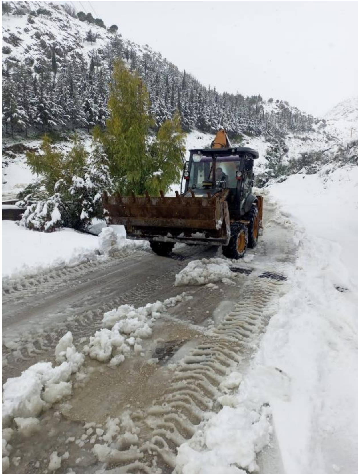
Road opening in Qab-Elias, Central Bekaa through a Save the Children supported project under Social Stability sector. Photo: © Qab-Elias Municipality
