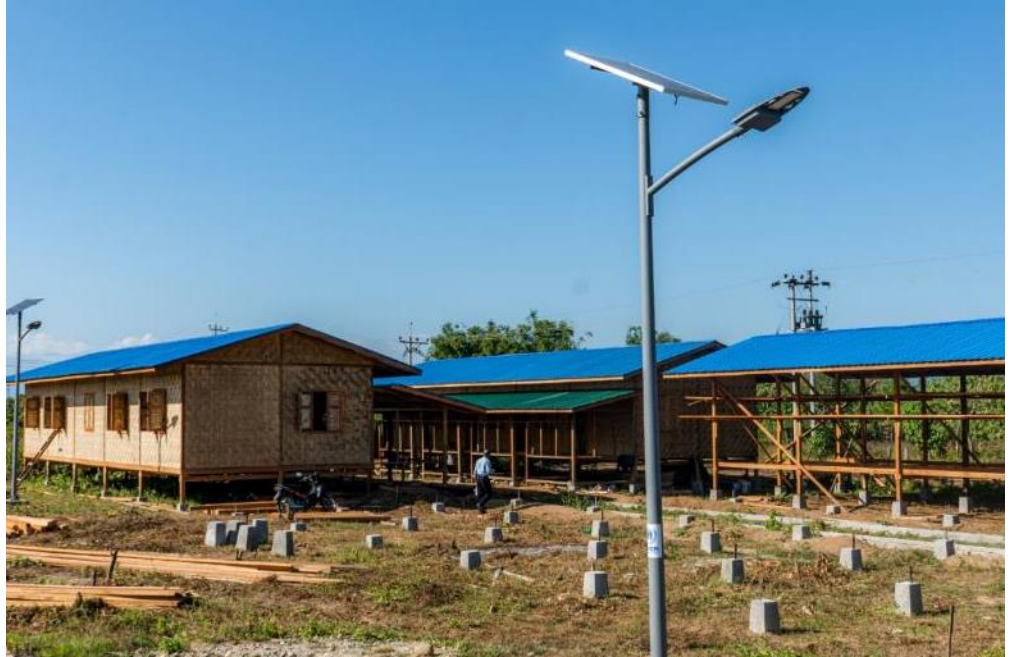
UNHCR provides targeted shelter support to IDPs in Kachin State. New homes are constructed for families and solar streetlights are installed to illuminate pathways and provide a sense of security. © UNHCR
