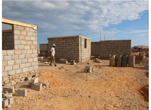
Construction of permanent shelters in Girible-2 Durable Solutions Site in Bossaso. © NRC \ Suleiman
