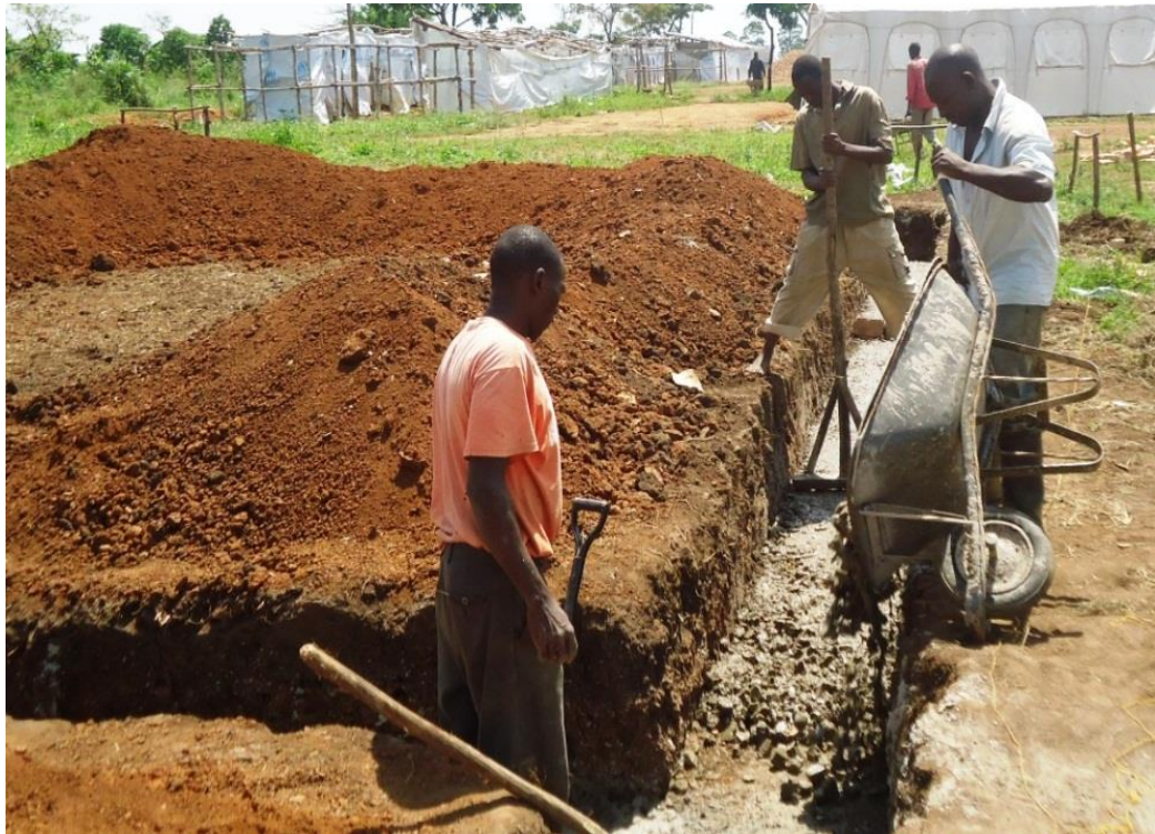
Construction work of a reception centre at Kagoma is underway in Kyangwali settlement. ©UNHCR/J.K. Lotweny
