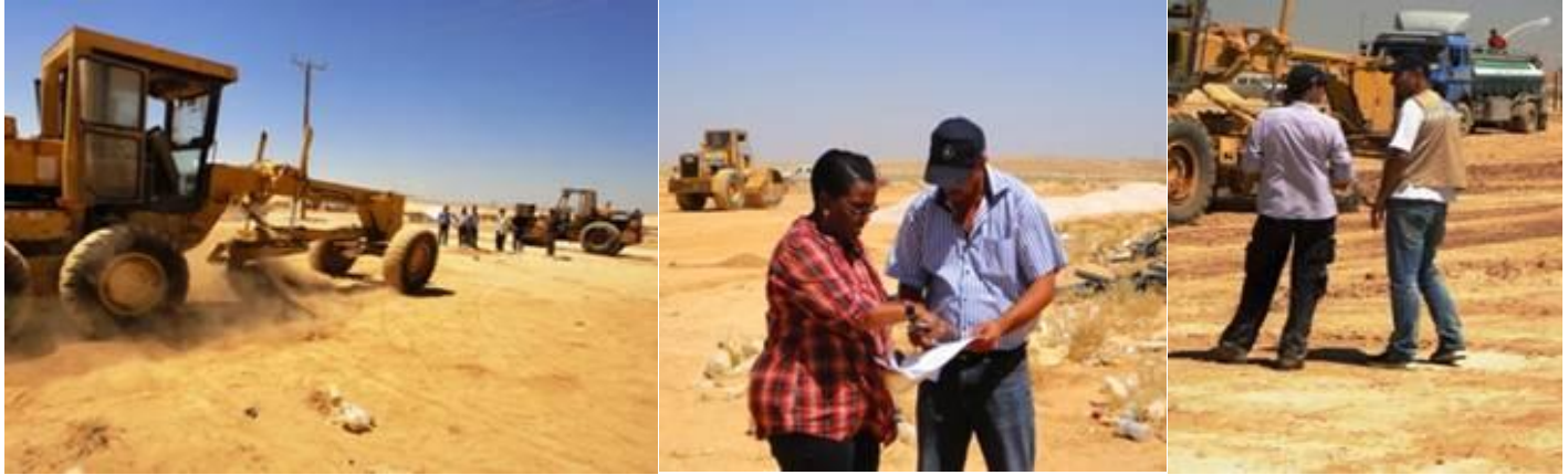
Construction of WFPs food distribution point in Al Zaatari Camp © WFP/ Dorte Jensen and Hani Abuarja
