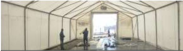
New flooring being installed in the Habitat for Humanity Rubb hall in the Vinojug reception centre. © UNHCR/H.Hababbeh Gevgelija (FYR Macedonia) 18 February
