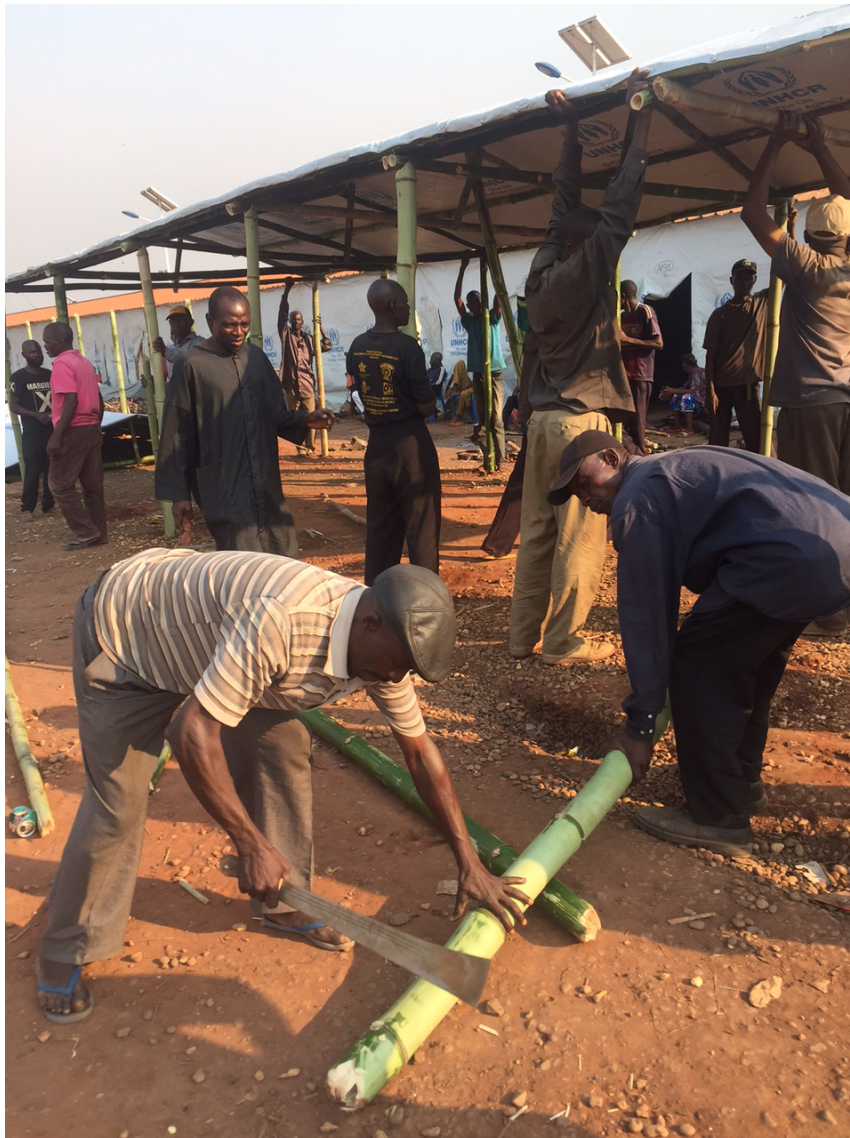
Refugee workers building hangars to shelter the expected arrivals at Cacanda reception centre. UNHCR / Katja Rytkonen.
