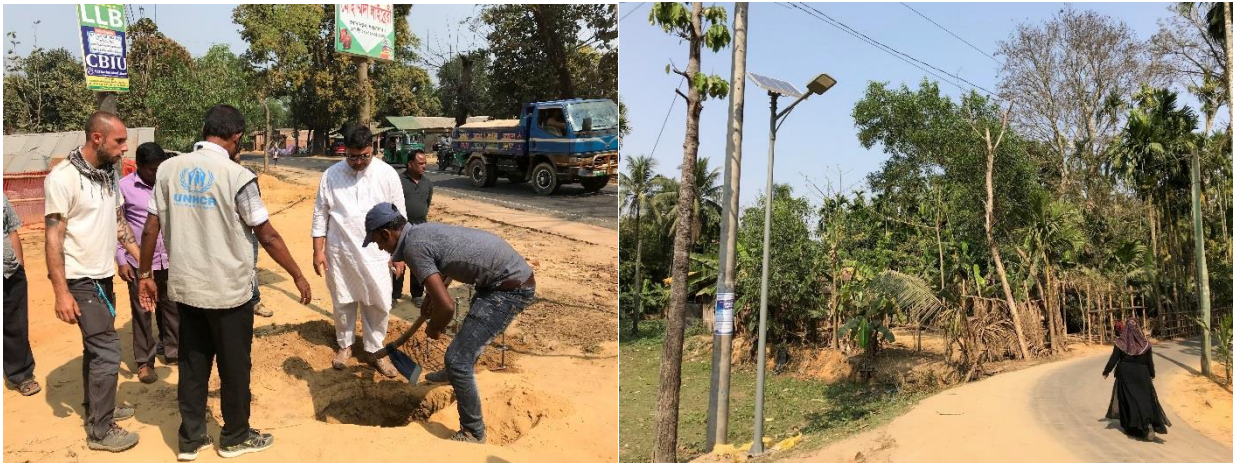
From left to right: Before and after photos showing a solar street light being installed in Foliapara village, located on the fringes of the giant Kutupalong Rohingya refugee settlement. © UNHCR/Caroline Gluck
