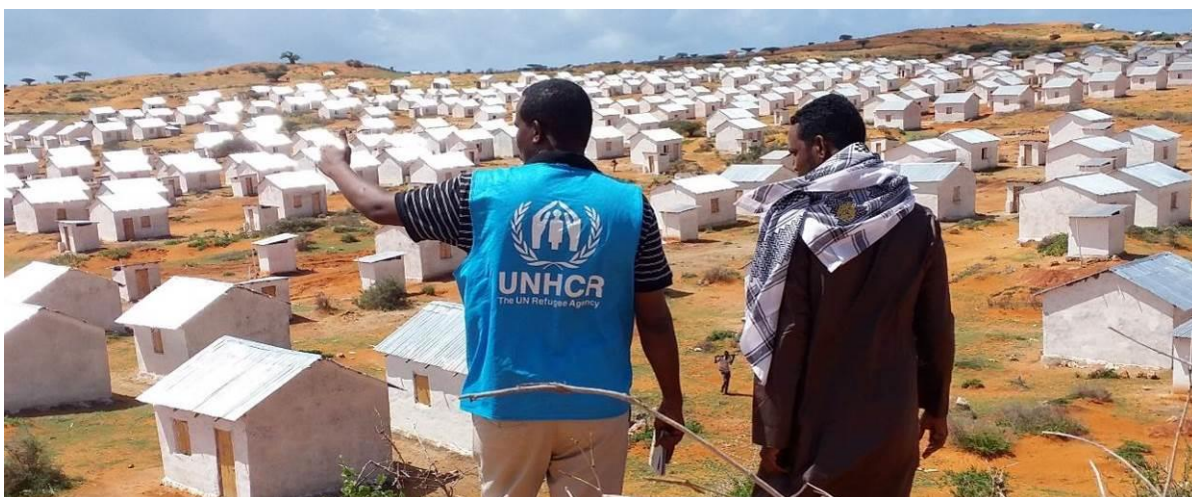
Constructed shelters and latrines in Kismayo will be a new home of returnees, IDPs and local community. © UNHCR/May 2017
