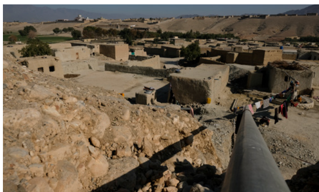
The 2,600-metre water pipe system runs down from the main water reservoir (which holds 60,000 litres of water) bringing vital water to a small village in Behsud District of Jalalabad. ©UNHCR 2017/S. Rich
