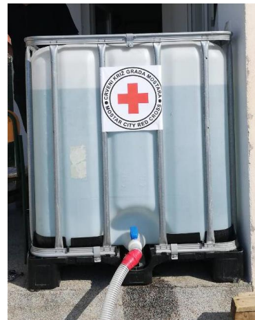
New 1,000 litre water storage tank at the RRC/Red Cross, August 2018
