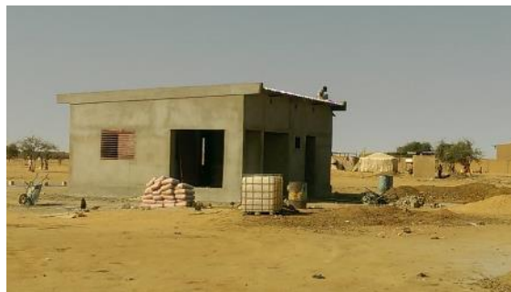
Construction of living quarters for doctor and midwife at Intikane health centre.
