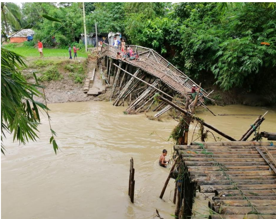
Due to heavy rains and wind, which resulted in flooding, refugees and host community were affected and displaced in the southern Teknaf region of Cox's Bazar. In addition to shelter damage, some of the bamboo bridges that enable mobility within the refugee camps were also damaged. Photo: ©UNHCR/Therik
