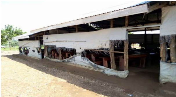
Dilapidated classroom at Ofua II Primary School to be upgraded
