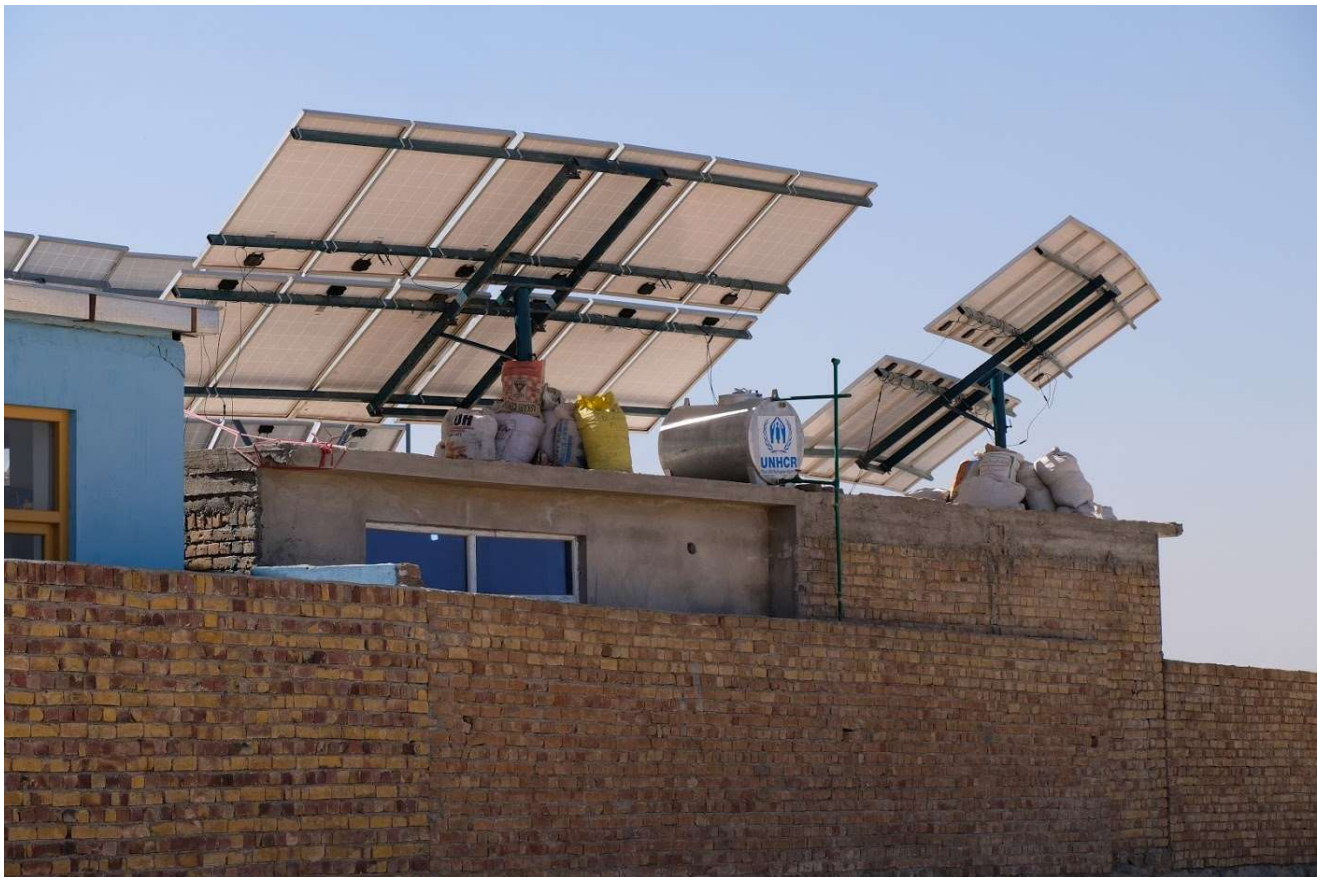
A UNHCR-constructed school in Tarakhail Daag, a priority area for return and reintegration in Kabul province, uses solar panels for electricity and water. UNHCR/H.Macdonald
