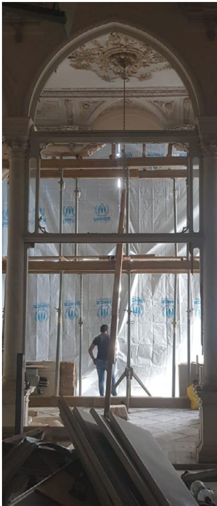
A heritage building is protected from the elements ahead of winter with plastic sheeting. Photo © BBHR
