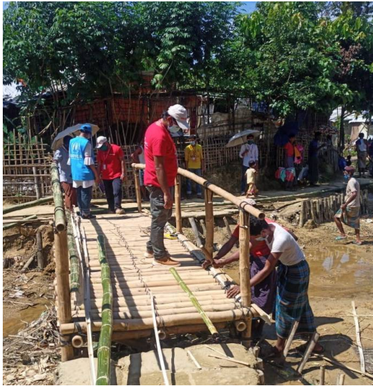
Labourers building a bridge, as one of the projects identified by community members in C21 through the ongoing community led projects © UNHCR/Rimi Akther
